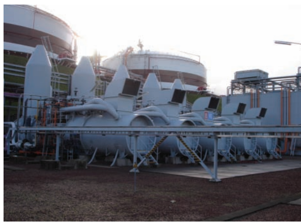
Picture 3: The LNG Peak Shaving installation has 5 LNG evaporators. In the background you can see the overground storage tanks.
